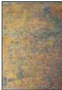
Figure 2.2: Uniform Corrosion (www.materialsengineer.com)
